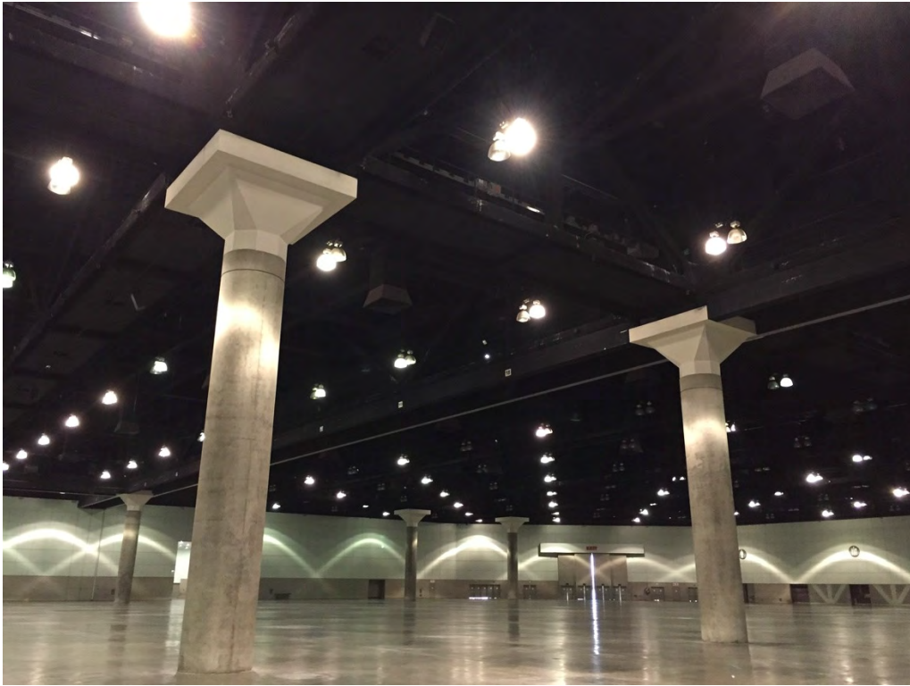
Figure 11: South Hall, main exhibition structure, showing steel columns (with concrete cover) and steel mega-trusses above.
