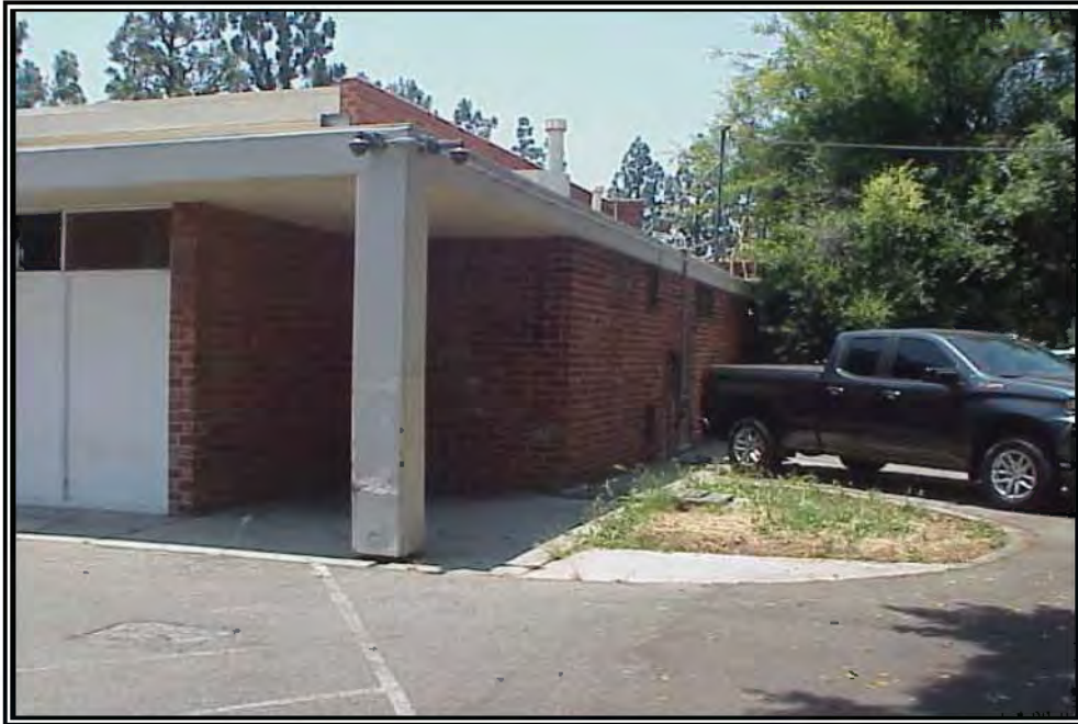
View of the north elevation of the subject property looking southwest from the northeast portion of the site
