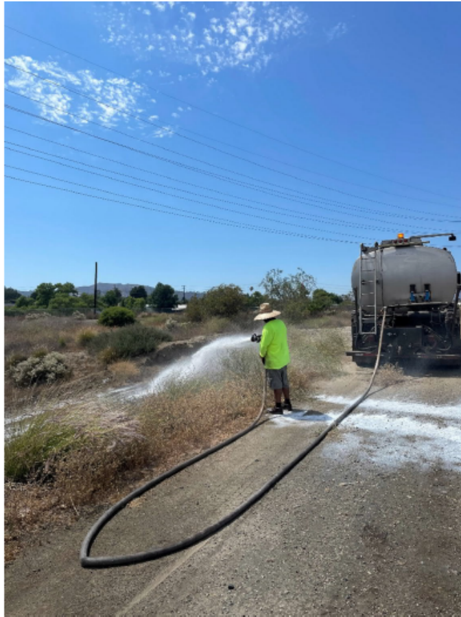
Dust suppressant application in former storm water basin adjacent to interior road closest to LA river channel
