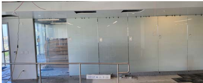
VIEW OF SMARTGLASS WALL (W/ TEST PANEL ON FAR LEFT, IN CLEAR MODE)
