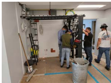
VIEW OF IT/ DATA ROOM
