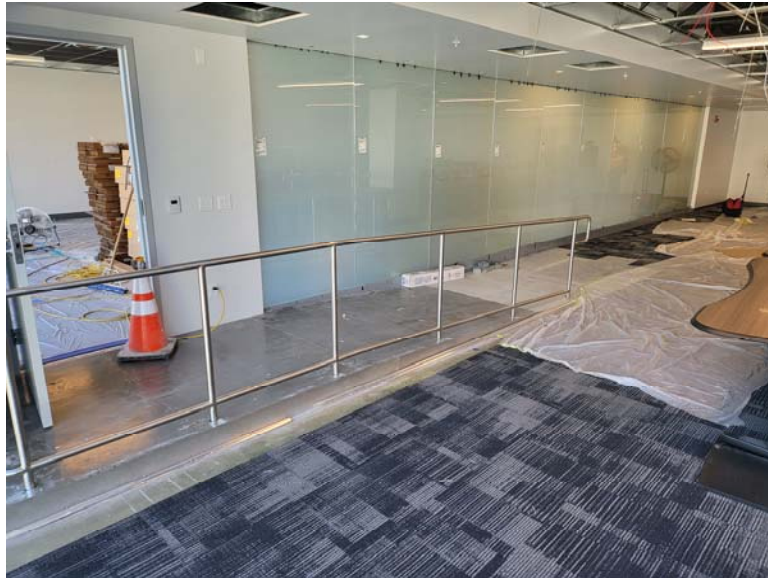
VIEW OF SMARTGLASS WALL SEPARATING THE CONTROL AND DEMO ROOMS (W/ SMARTGLASS IN OBSCURE MODE)
