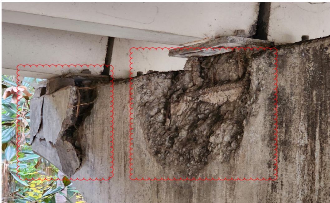
Spalls With Exposed Rebars on the North Pier
