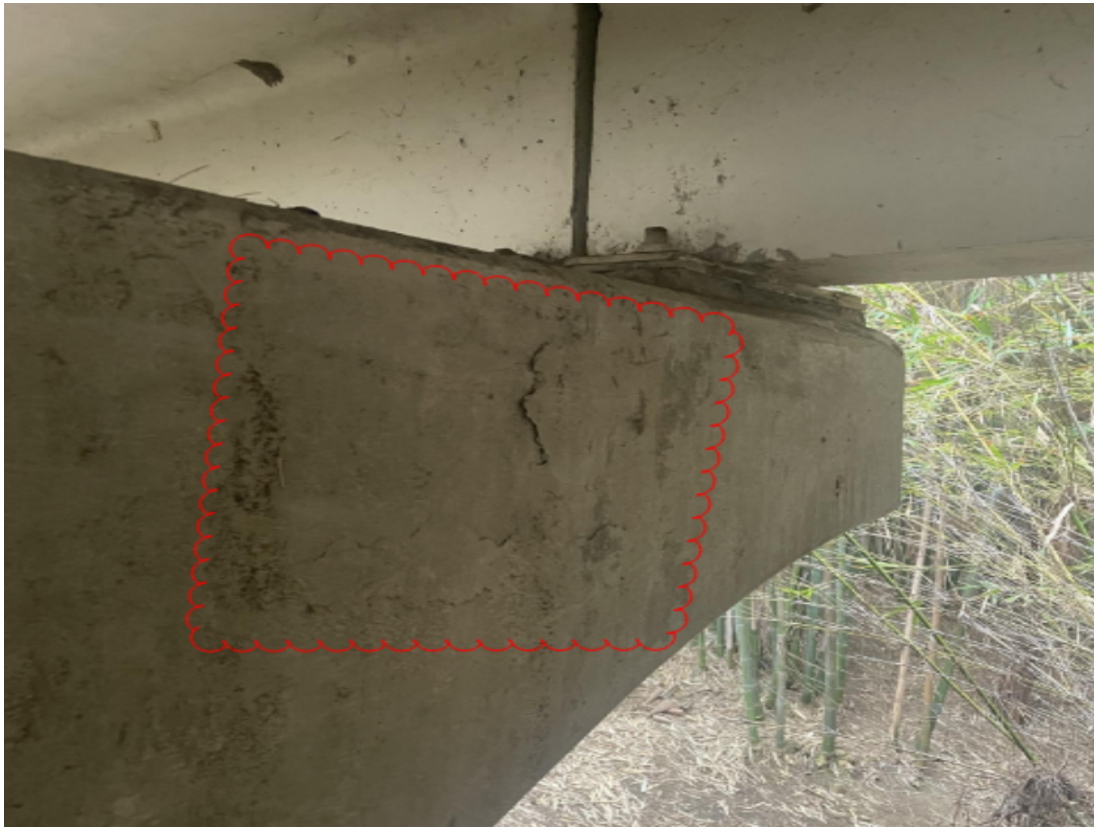
Minor Spalls on the South Pier
