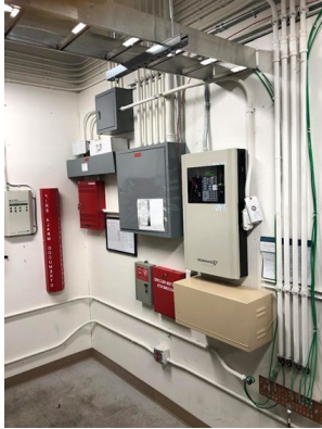
LAPD Topanga Station New Fire Alarm System
