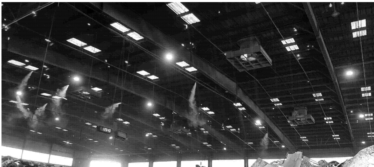
Figure No. 1: Current Roof Condition at CLARTS Transfer Building
