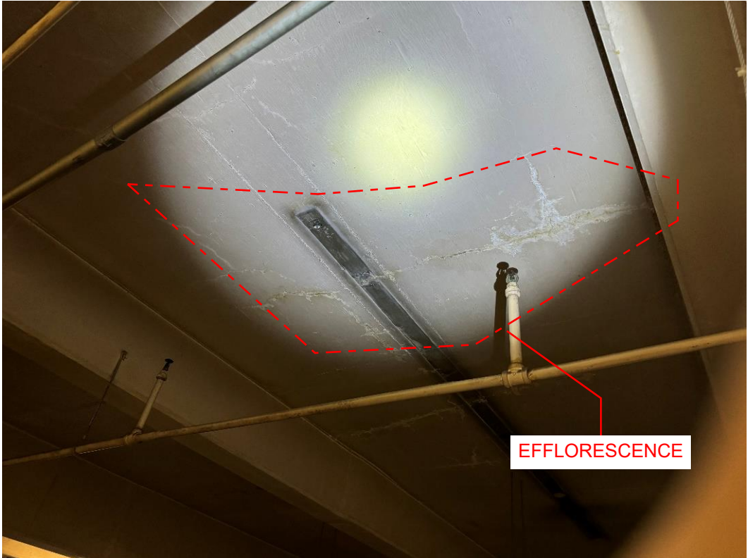
Photo 11: Efflorescence in Soffit Slab
