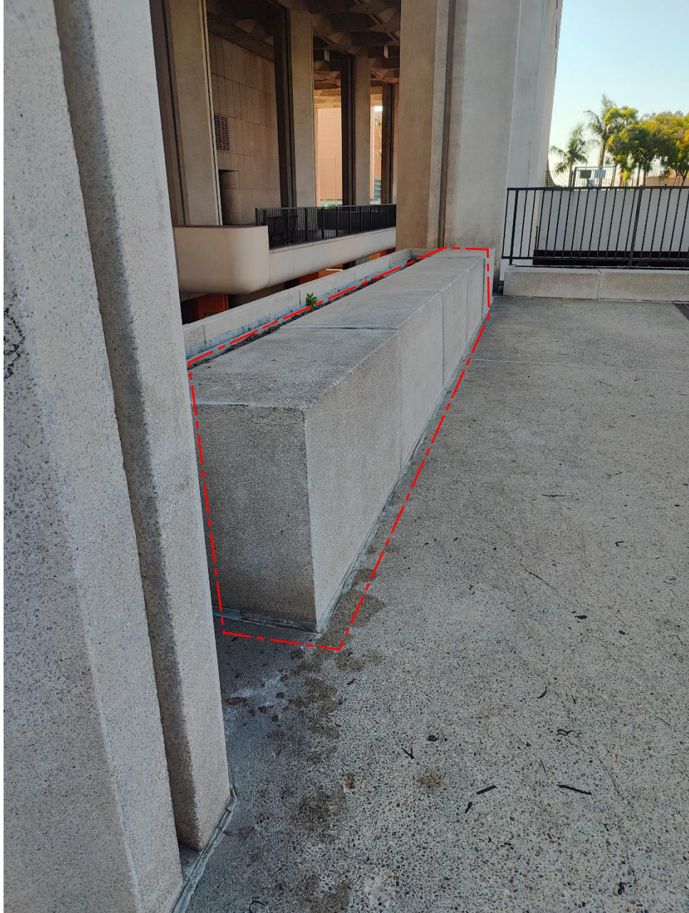
Photo 17: Contorted Parapet/Planter Wall
