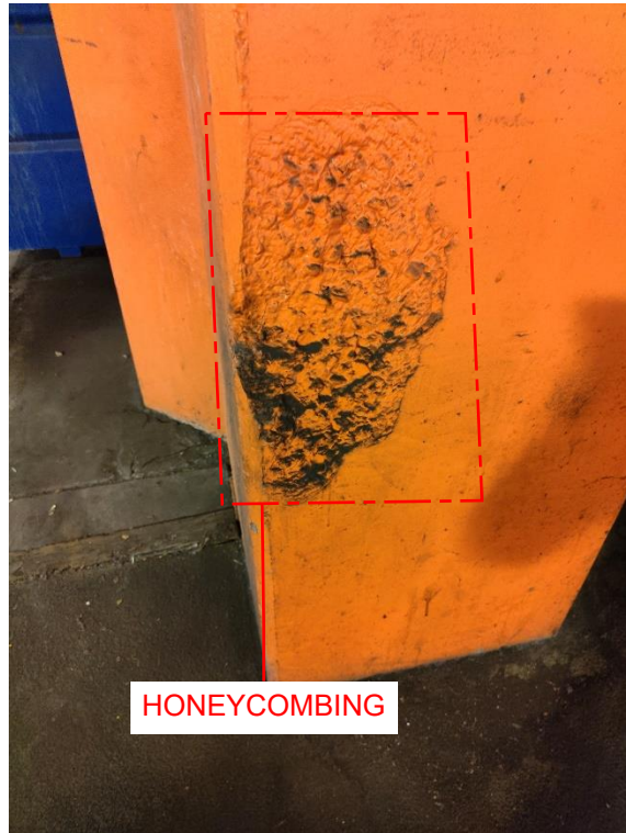
Photo 15: Honeycombing at F-2 Column
