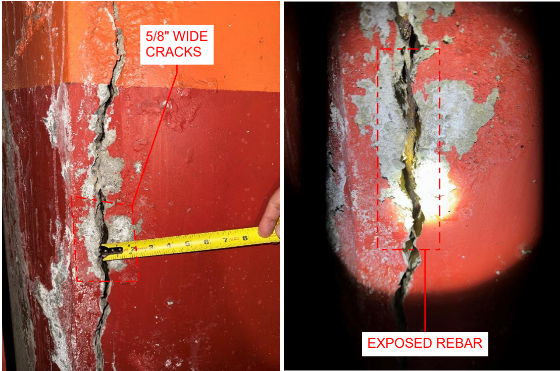
Photo 14: Column Corrosion Cracks
