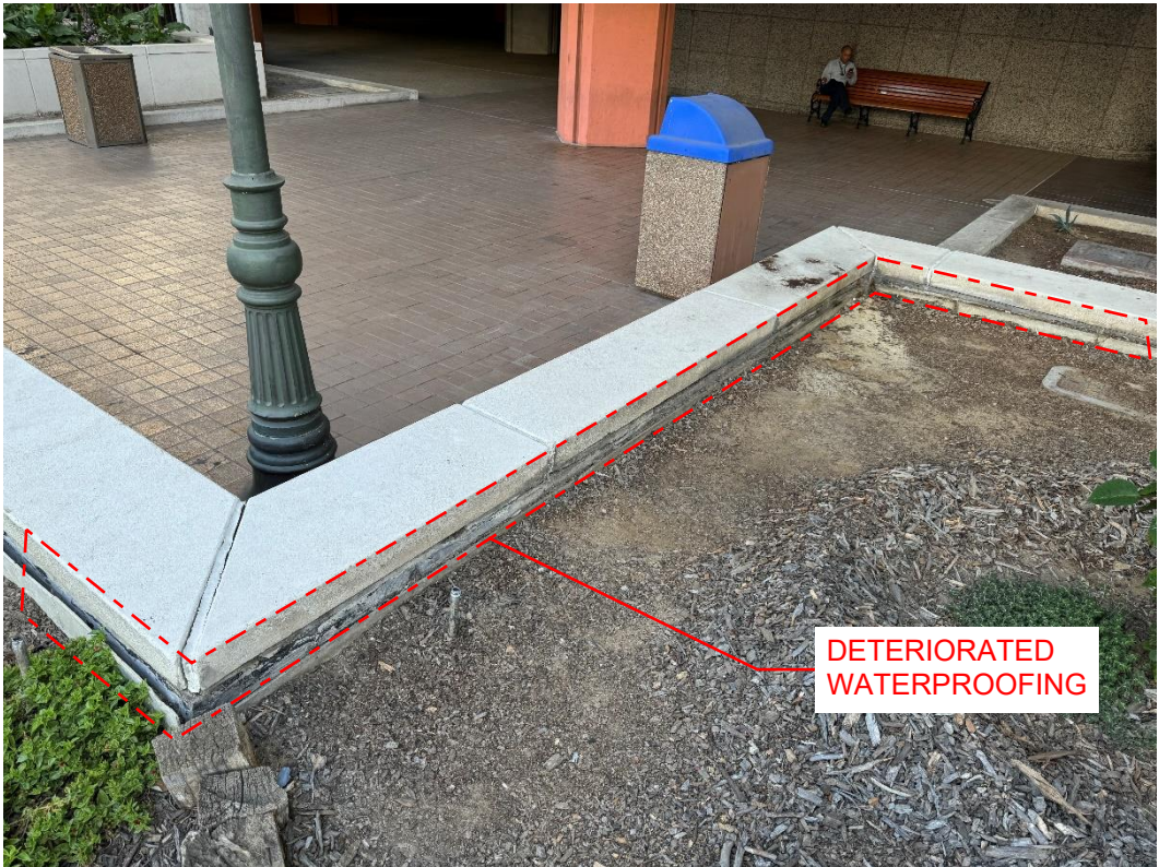
Photo 7: Deteriorated Waterproofing at Planter Walls
